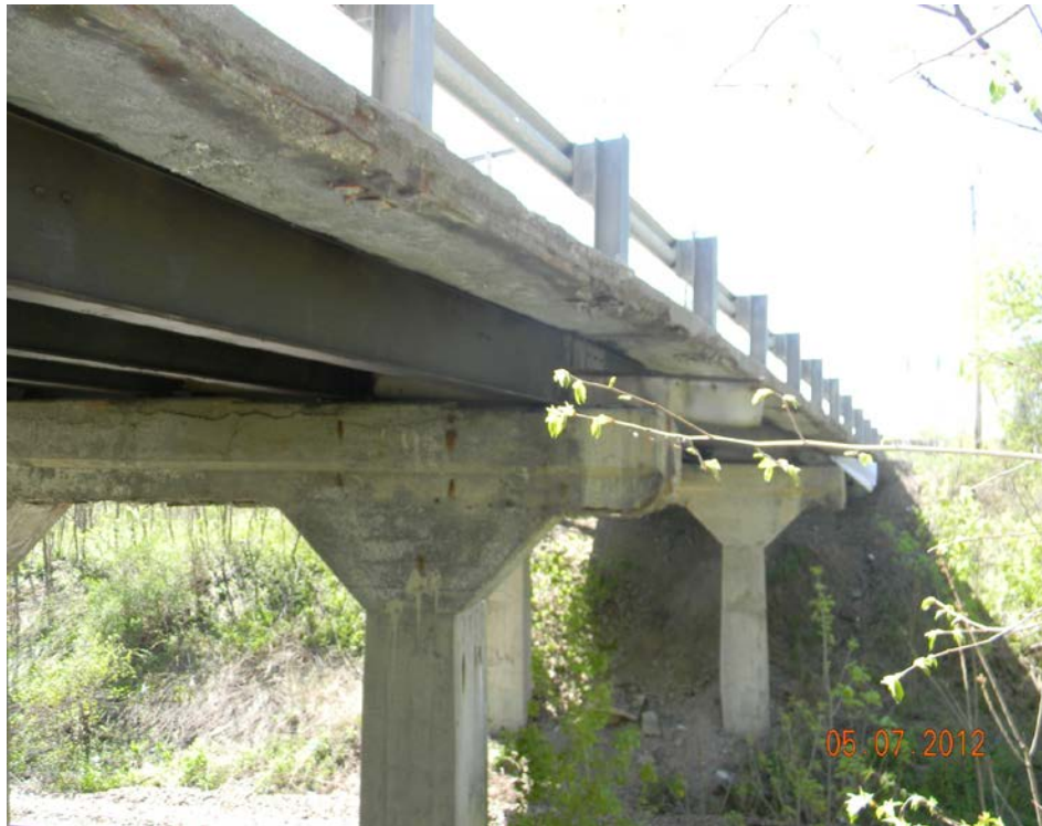
East side of bridge looking north – Deteriorating Deck Overhang
