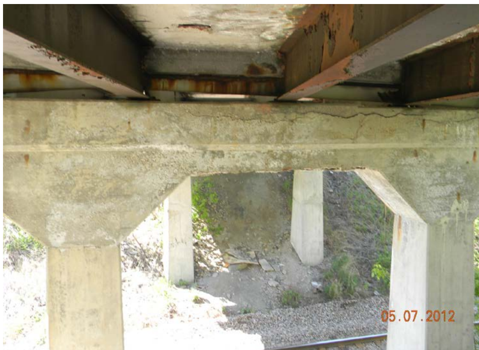
Underside of bridge looking north – Deteriorating Superstructure
